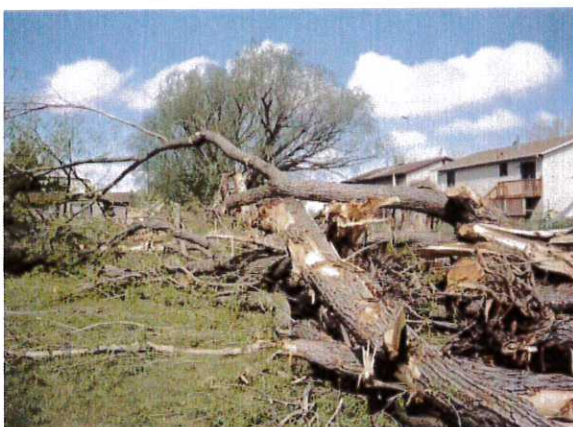
In the summer of 2004, volunteers removed the trees, laid a pipe in the ditch and leveled field.
